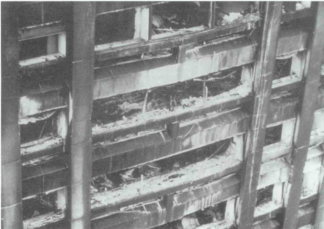
◀ The charred exterior of One Meridian Plaza in Philadelphia following the March 23, 1991 fire.
